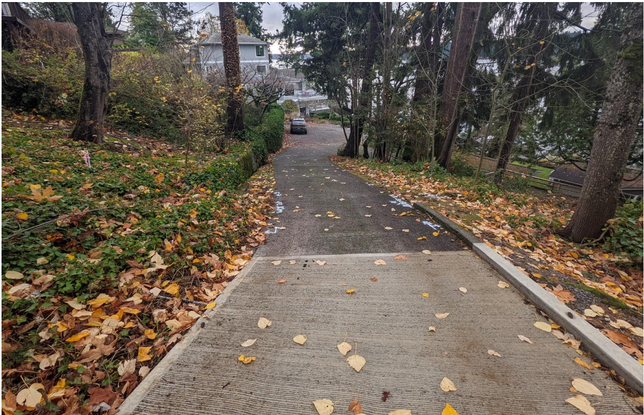
Plate 5. General conditions of the shared driveway in the eastern (upper) portion of the site, looking west.
